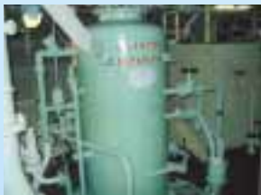
Oily Water Separator
